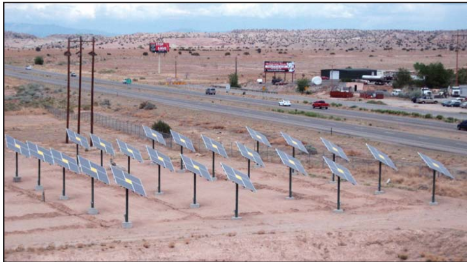
■ UniRac designed and manufactured a custom sunflower poletop rack for PNM's high visibility installation adjacent to Interstate 25.
