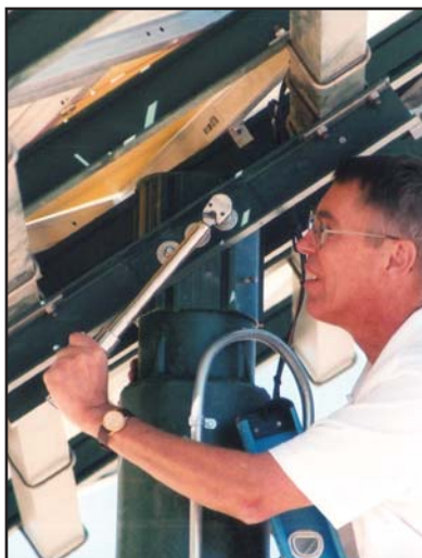
■ Phil Crosby, UniRac's Product Development Manager, tests torque at the installation site.
